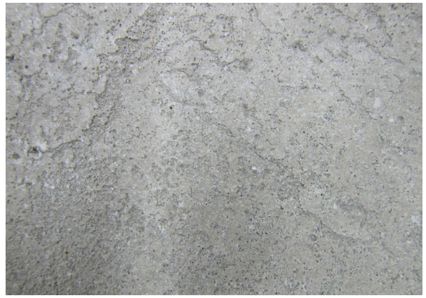
(c) Surface Deterioration after 25Cycles of Scaling Test
