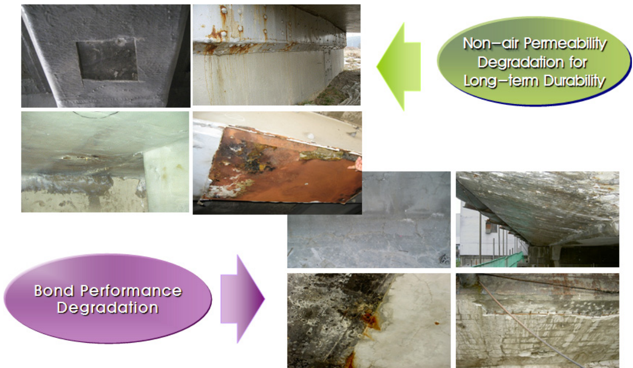
Fig. 1 The field victimized case of the structure reinforced by the steel plate pressing process
