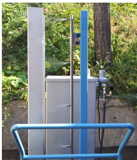
Fig. 7 General view of a utility system for cleaning
