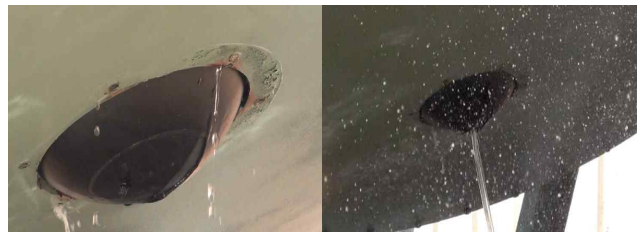
Fig. 15 Rupture and leakage of 200mm puncture under pressure of 0.7bar
