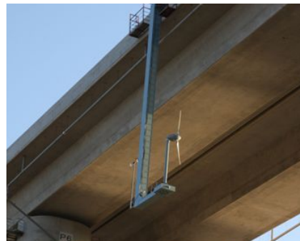
Fig. 1 Installed wind turbine, Skystream 3.7
