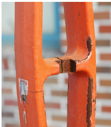
Fig. 20 Gap Part Corroded
