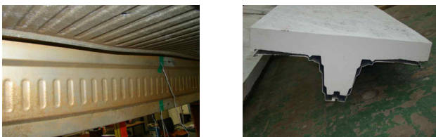
(a) Deck bending deformation (b) Bond failure Fig. 8 Fracture mode of specimens (SCS200-1.0R)
