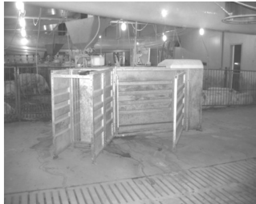
ESF installed in pen
