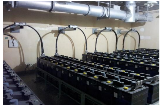
Fig. 3. Battery room in nuclear power plant
