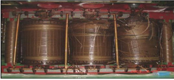
Fig. 3. Damaged three phase step-up transformer
