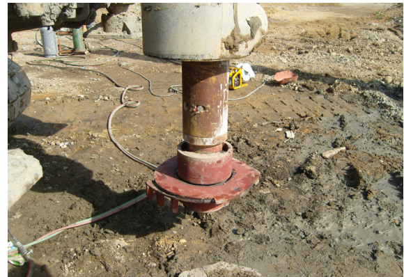
(a) Pile Toe (b) Bottom shoe Fig. 4. The toe-jetting shoe type construction method
