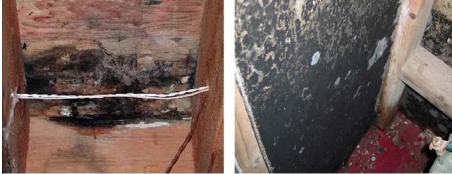
Fig. 2. Outbreak of black mould by thermal bridge[5].
