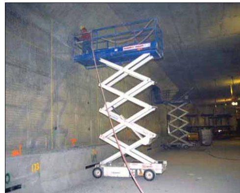
Figure 2. An example of working on a motorized lifting platform in construction industry
