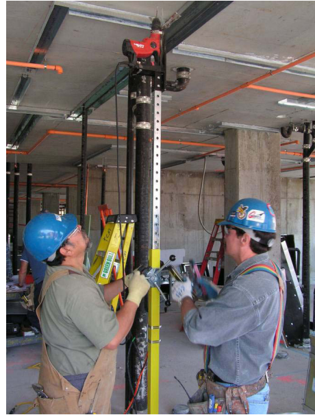
Figure 1. Inverted drill press intervention design using a rotating handle and linear gear to raise the inner (silver) column
