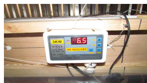
(b) Heating cable thermostat
