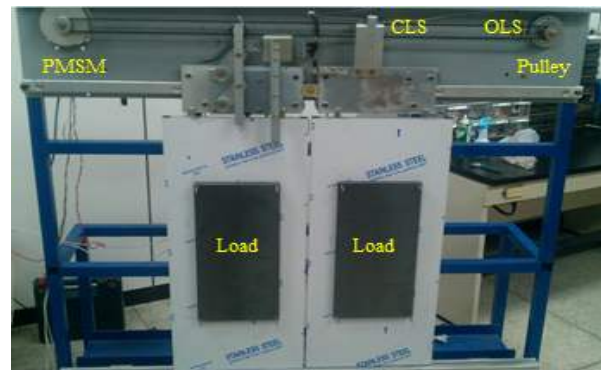
Fig. 9 Experimental setup for elevator door speed control
