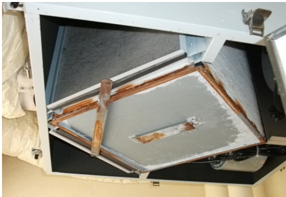
Fig. 1 Corrosion of a heat recovery ventilator by dew condensation.
