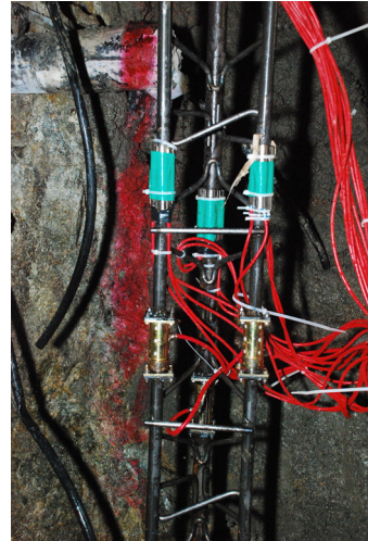
Fig. 9. Load cells and vibration wire strain gauges installed in the lattice girder
