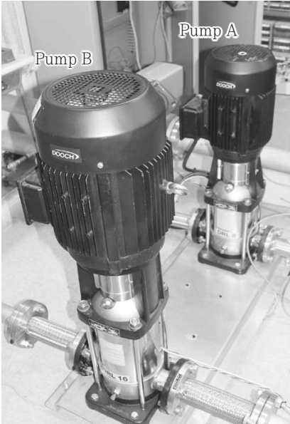
Fig. 9 Photo of Pump A and B
