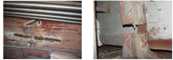
Fig. 1 Crack and fatigue damage in transition zone
