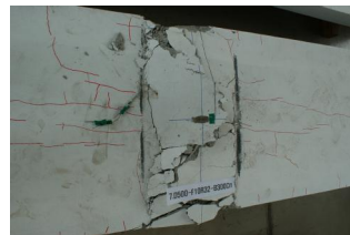
Fig. 13 Failure shape : no bottom rebar
