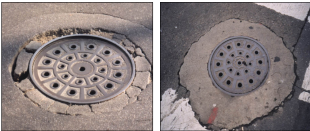
Fig. 1 Patterns around the damaged manhole
