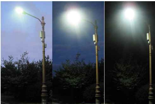
(a) 50% lighting (b) 70% lighting (c)100% lighting
