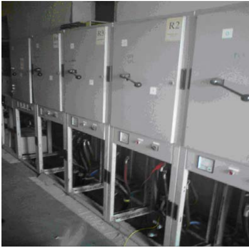
Fig. 7. Working environment in transformer station 10/0.4 kV.
