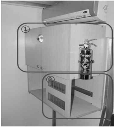
Fig. 12. Outside of Cabinet
