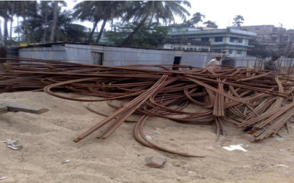
FIGURE XVI WRONG MANAGEMENT OF STEEL AT MUSLIM SAHIYA SANGSAD PROJECT.
