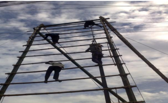
FIGURE XVII UNCONSCIOUSNESS OF WORKERS ABOUT SAFETY AT RIDGE TOWER IN DARGAH GATE.
