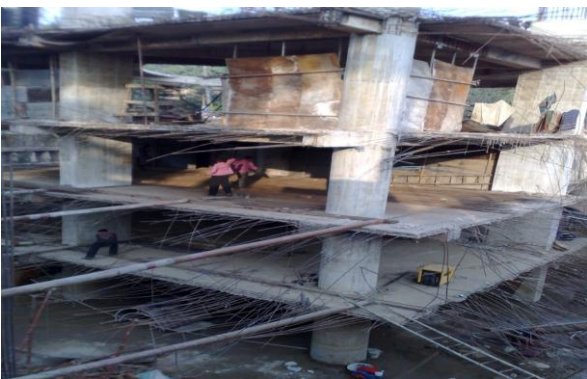
FIGURE XXV 3- SUB BASEMENT BELOW GROUND LEVEL WHICH IS VULNERABLE FOR EQ AT PUMP TOWER
