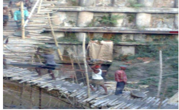
FIGURE XIX WORKER WITHOUT ANY SAFETY MEASURES AT ARK HOMES IN HAWAPARA.
