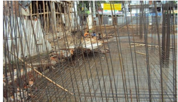
FIGURE XX SIDE WALL HAS BROKEN ON THE FOUNDATION AT MUSTOBA TOWER.
