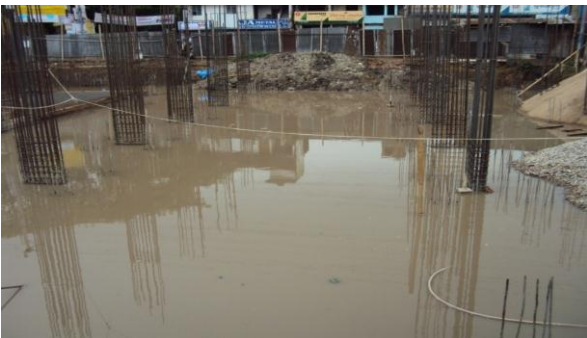
FIGURE XXIV FOUNDATION HAS FLOODED AT MUSTOBA TOWER IN ZINDABAZAR
