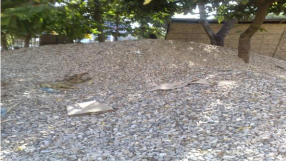
FIGURE XV THE COARSE AGGREGATES ARE GETTING MIXED WITH FOREIGN MATERIALS AT MUSLIM SAHIYA SANGSAD PROJECT.
