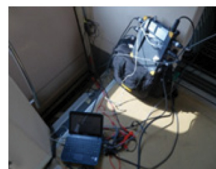
(c) PQM Equipment Connection
