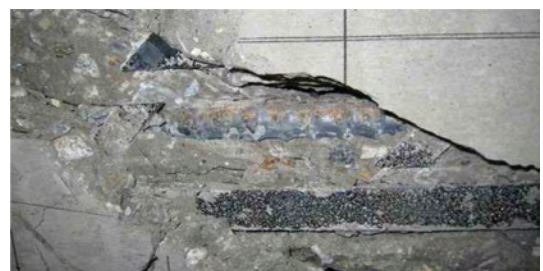
Fig. 5 Fracture of GFRP plates
