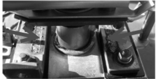
Figure 8: Arc damage of mechanical contactor
