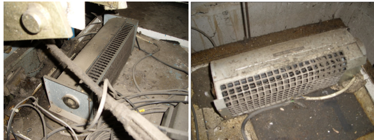
Fig. 3. The polluted elevator fan.
