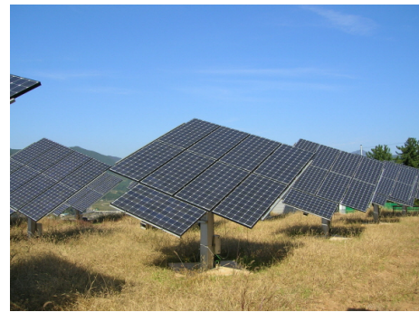
Fig. 7. PV array composition
