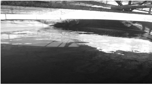
Fig. 19. Slurry mixing without air supply.
