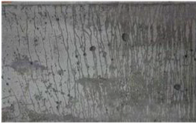
Fig. 12 Multiple micro cracks observed in specimen (Mix B2)
