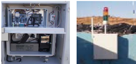
Fig. 3. Interior and exterior of sensor logger system.
