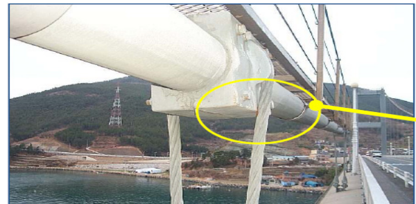
(b) corrosion in the contact area of hanger
