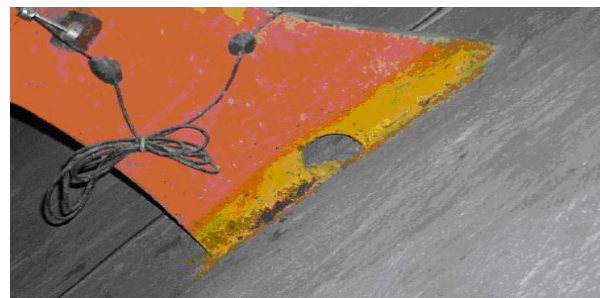
(c) corroded anchor bar in anchorage block
