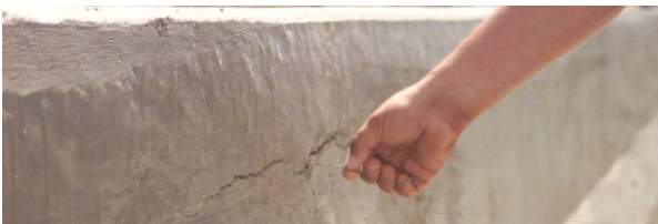
Fig. 2 Crack in Barrier
