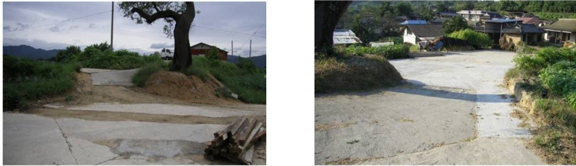
[Figure 3] Examples of improvement 2 Left: Repair of road pavement done by farmers. Right: After improvement.
