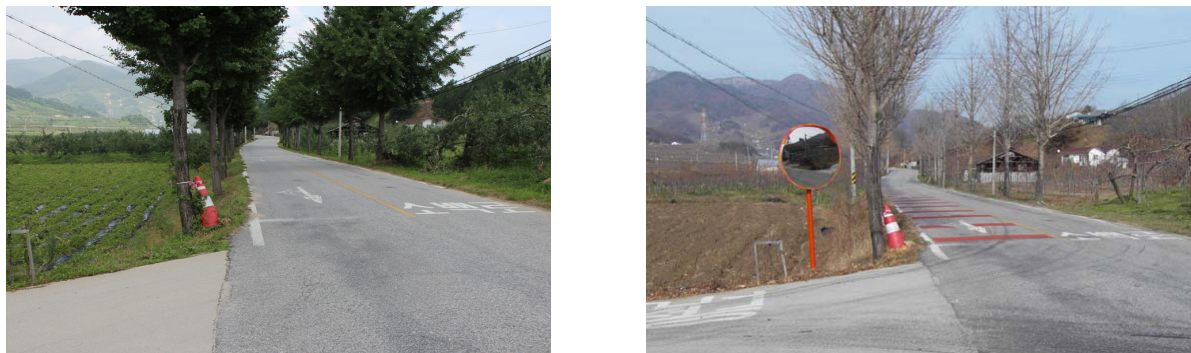
[Figure 4] Examples of improvement 3 Left: Road reflector and speed reducing bump. Right: After improvement.
