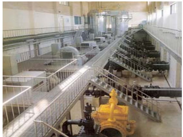
Fig. 2 Picture of Juam intake pumping station(1st stage)
