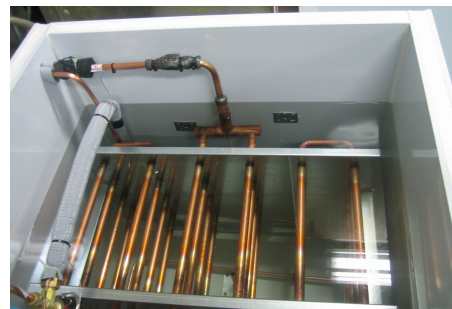
Fig. 2 The inner of cold-thermal storage tank
