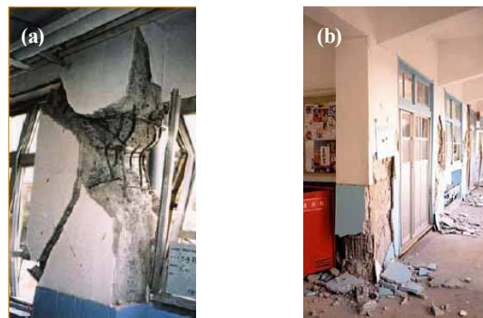
Fig. 1. RC column failure of school structure:(a) shear failure and (b) flexural failure[13]
