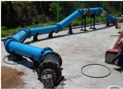
Figure 10: 3-D pipeline for experiments
