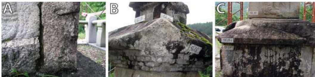
Fig. 5. Physical weathering of the pagoda. (A) Exfoliation of basement rocks (B) Broken stones (C) Cement mortar of the basement stones.
