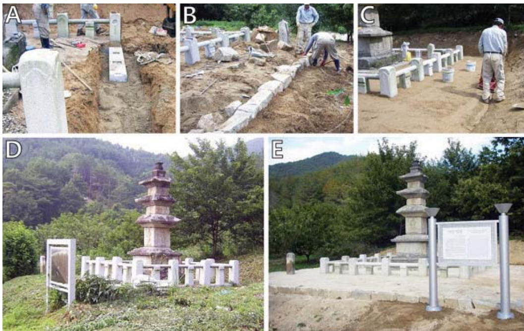
Fig. 9. Protective railings reinstallation(A), site rearrangement(B, C) and before and after the treatment(D, E)
