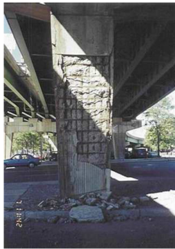
4 th Deterioration Stage Inspection Year = 2000
