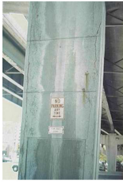
2 nd Deterioration Stage Inspection Year = 1988
