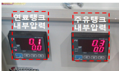
Fig. 6 Tank Pressure before Refueling
