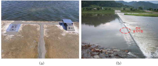
Fig. 9. Photograph of the Acoustic Profilers Installed on the Crest of Songdong Weir (a) and Flow over It (b)
