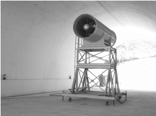
Fig. 5 Photograph of jet fan
