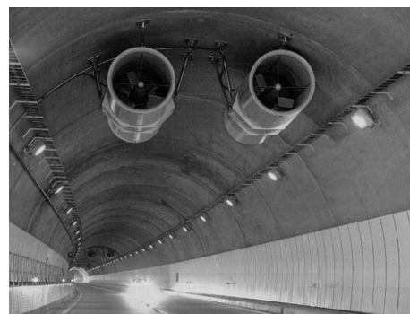
Fig. 2 Jet fans in parallel installed in road tunnel
