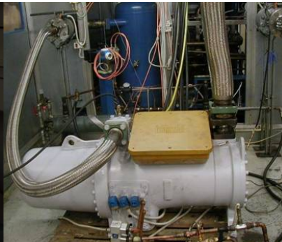
Fig. 7 Refrigeration compressor, Broglia, 2007
