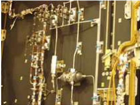
Fig. 12 Test Section of Pressure Regulator
