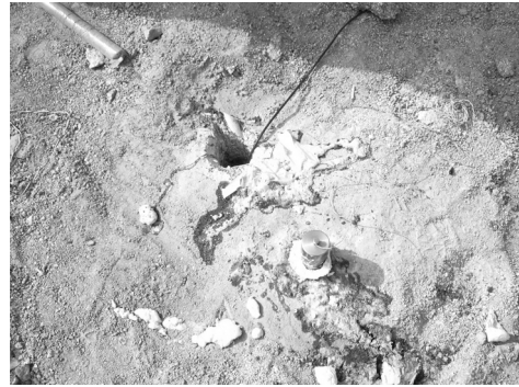
Fig. 6. The sensor appearance inserted into the bore hole.
