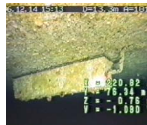
Fig. 2. Sacrificial Anode, Clean
