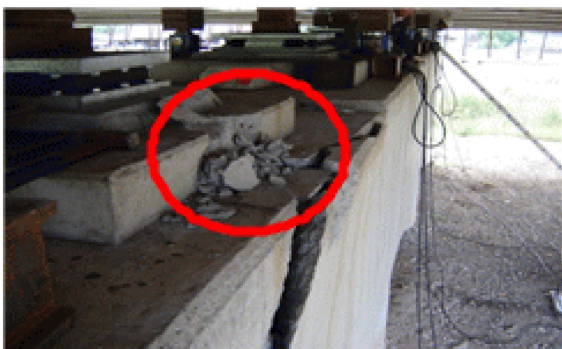
Fig. 4. Damaged concrete of shoe support.
