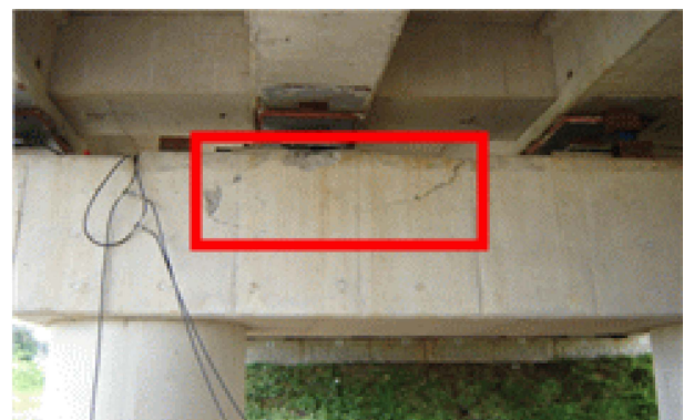
Fig. 1. Front view of damaged concrete pier.
