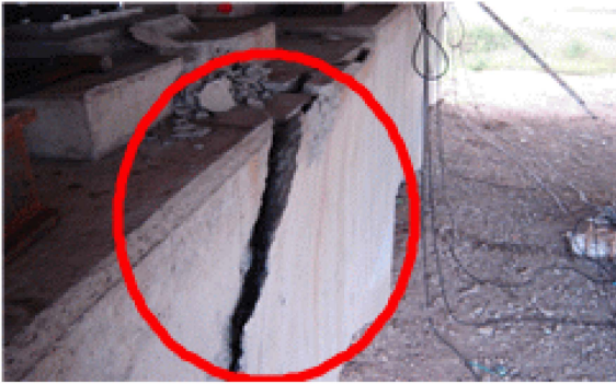
Fig. 2. Detail panorama of damaged concrete pier.
