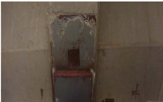
Fig. 3. Detail view of damaged concrete pier after cutting.
